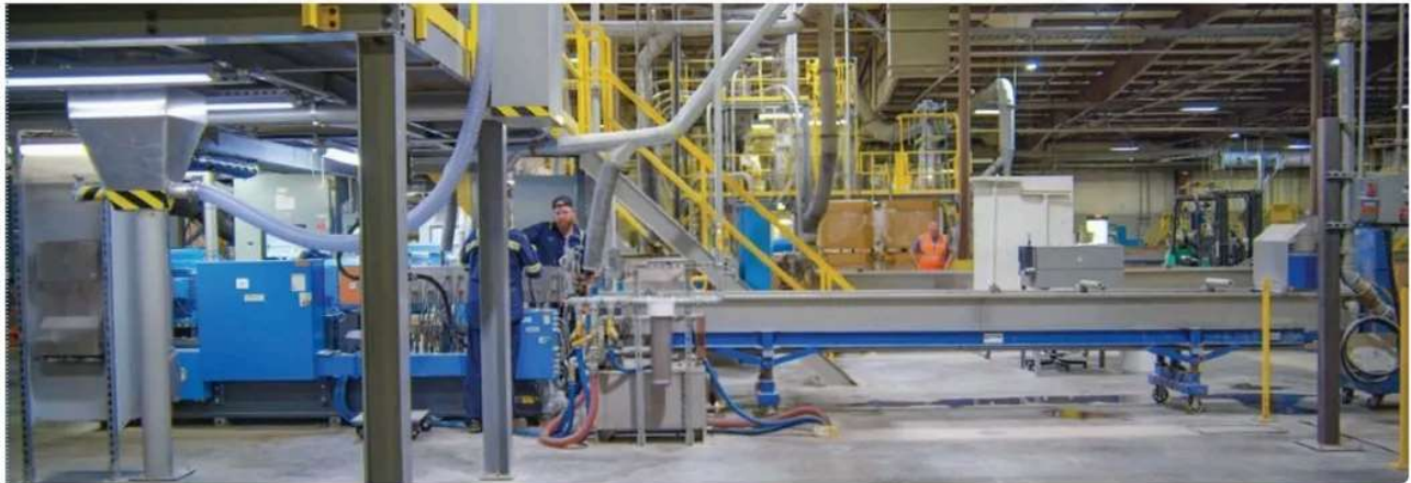
Star Plastics saw marked improvements in throughput and flexibility after upgrading its extrusion systems, a project that included this new twin screw line from Coperion.
